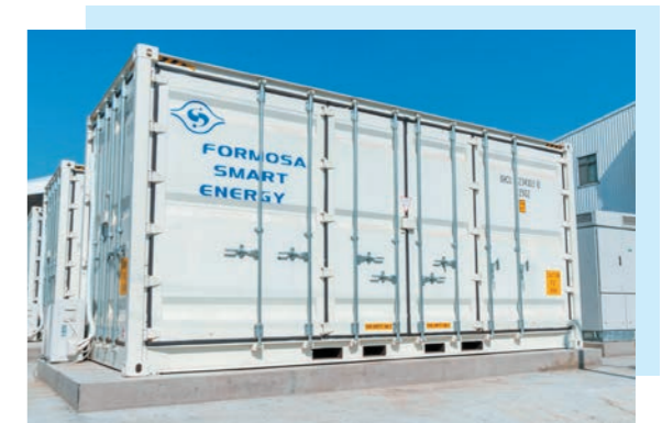
Formosa Smart Energy Tech Corporation - Energy storage system
