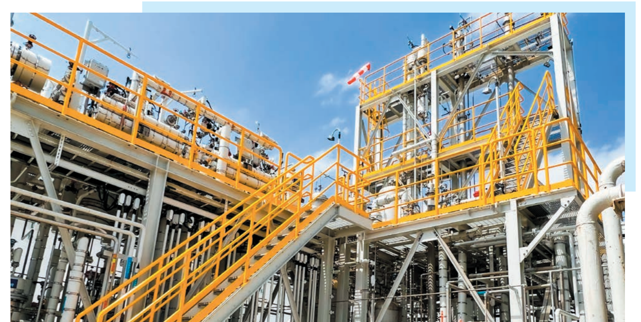
..... FPC Flue Gas CO 2 Capturing and Utilization Pilot Plant
